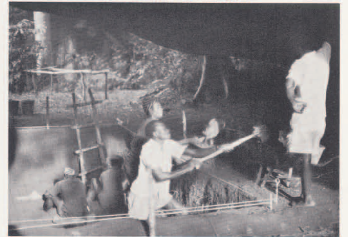
Work in progress: two men policing excavation of earth by hand; clean soil being loaded on a wheelbarrow.
